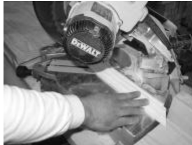
17) Using miter saw, cut base trim pieces to fit around bottom of column
