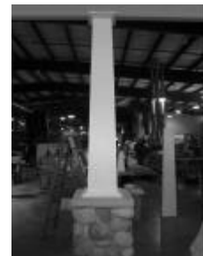
21) Clean surface of column with cleaner recommended by the paint manufacturer. Paint with 2 coats of acrylic latex paint.
