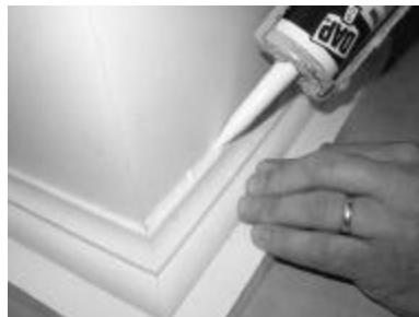
20) Caulk using latex caulking compound to fill an gaps & nail or screw holes.
