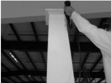
16) Glue 1/4 cap piece and slide into place. Pin nail cap moulding to top of column.*
