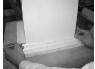
18) Use column shaft to mark cut lines for miters (cut long and work your way shorter for best results)
